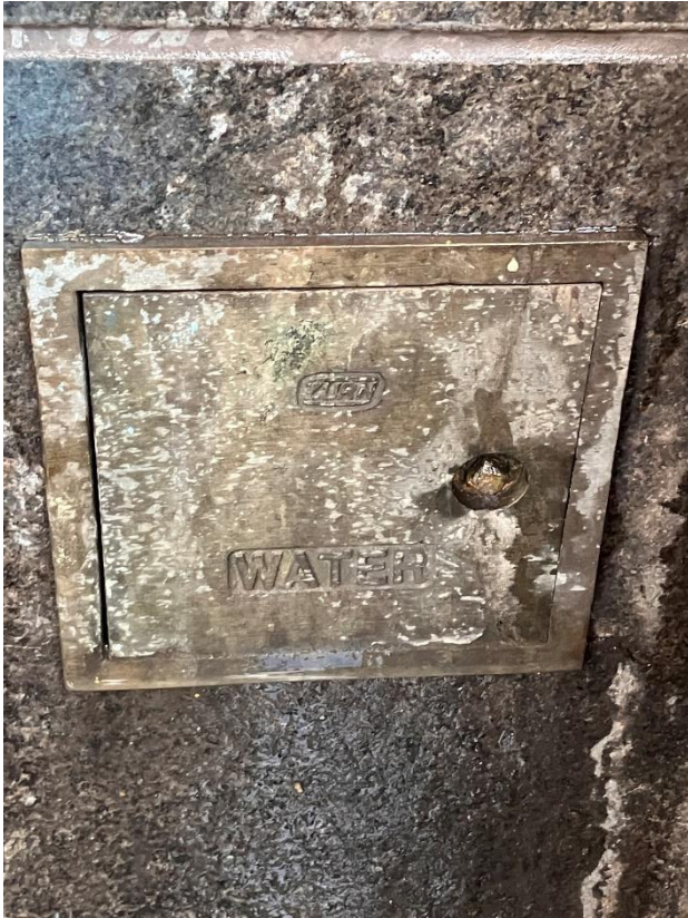
Close up of the box, clearly labeled "WATER."
